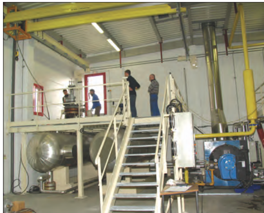
Steam test facility
