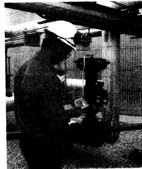
Figure 8.8. Two-way communication link with a digital positioner. (Courtesy of Fisher Controls International, Inc.)
