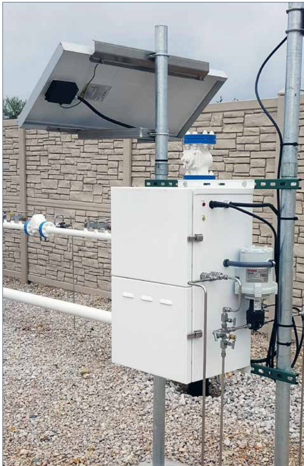
PAX 1 installed on a solar powered remote pressure control station.
